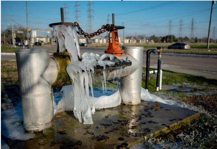
Valve Packing Leak
