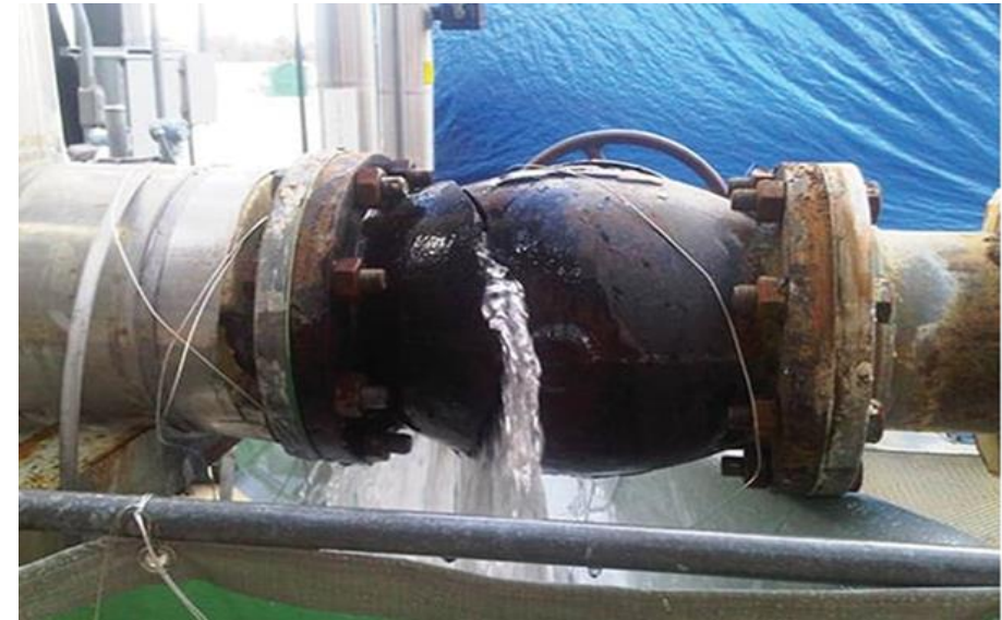
Valve failure due to missing insulation and heat trace
