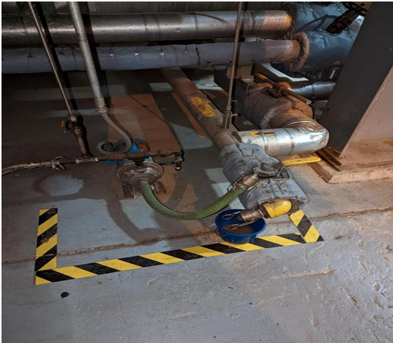
Offline Boiler Recirculation Pump
