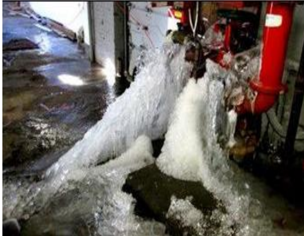
Frozen Fire Protection in unheated stair well
