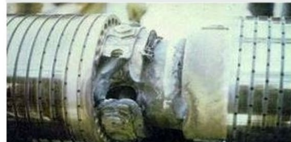
Catastrophic generator damage
